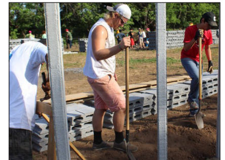
Construction workers from one of the mission teams this year helping to build the perimeter wall in Nagarote, Nicaragua.
