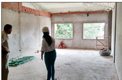
Frosty Hansen meeting with the architect on site at the future training center
